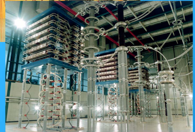
Pole1 refurbished with thyristor valves -1992
