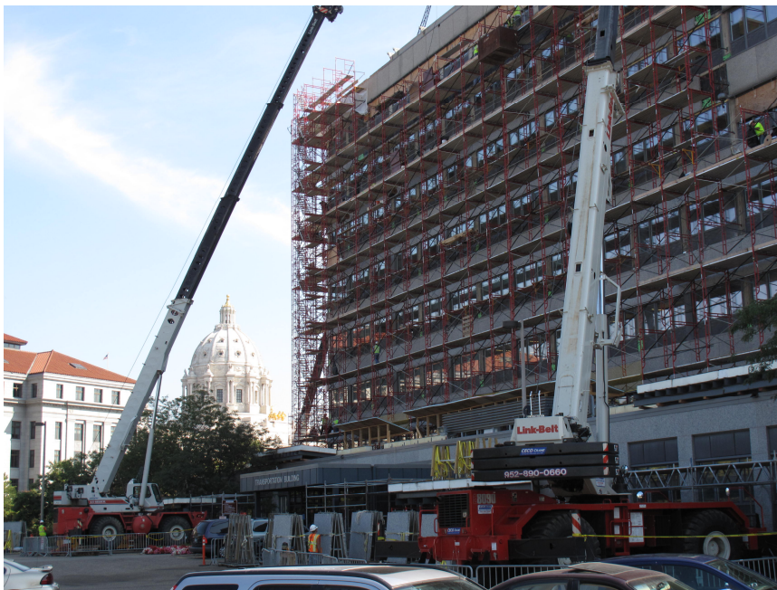
State of Minnesota – Transportation Building under construction (Photo by the author, September 2009)
